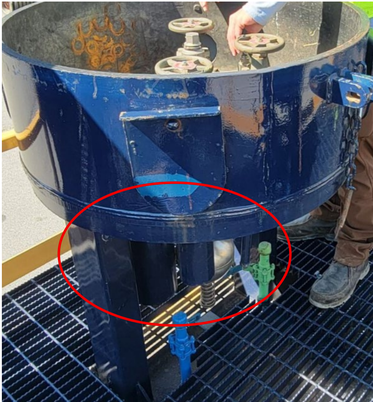
Exhibit I: Components under DOT112 prop show pipes and magnetic gauging device
